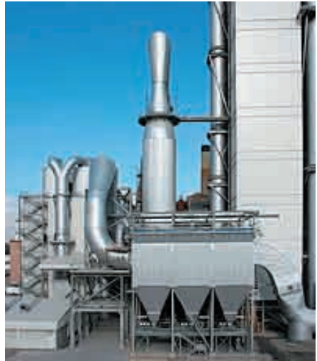
Castle Cement's filter and cooling tower at Padeswood. Dioxins and Furans may be produced when exhaust gases cool, and cooling these gases quickly through the critical temperature range of 450 to 200°C has been demonstrated to reduce dioxin and furan formation in cement kilns [Commission for Environmental Co-operation, p. 60]. Picture from www.castleceement.co.uk .
